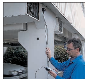
Measure air velocity with the large vane, e.g. at duct exits
